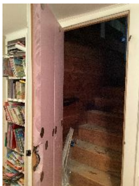
#9 – The door to the attic is well insulated, continuing the thermal boundary between the living space and the attic.
