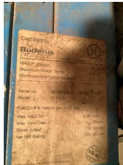
#5 - The serial number of the hot water heater suggests the boiler was manufactured in 2009.
