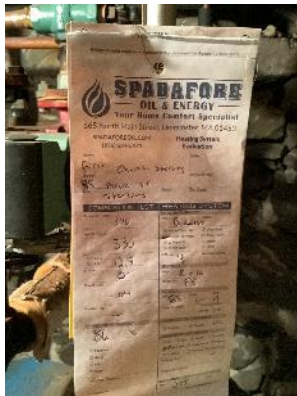
#2 - The service tag on the boiler shows it received regular maintenance. Good work!
