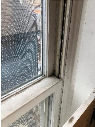
#7 – The Parsonage windows are double pane replacements, believed to have been installed as part of the 2014 renovation.
