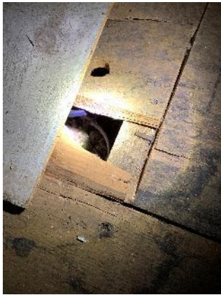
#8 – Blown in cellulose insulation has been added to the attic floor, as shown by the hole drilled into the floor board and the material seen in the gap between the boards.
