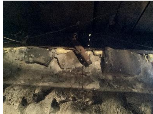
#10 – Spray foam has been applied to seal areas between the stone foundation and the wooden floor framing members. This reduces cold air infiltration – as well as mice and insect intrusions!
