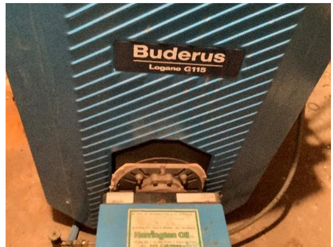
#4 - The oil-fired Buderus boiler is about 85% efficient.
