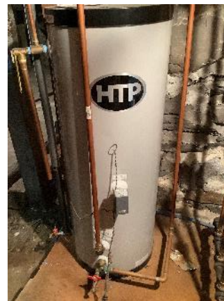
#6 - The hot water tank is an indirect model, circulating hot water from the boiler through a heat exchanger. Note the uninsulated pipes.
