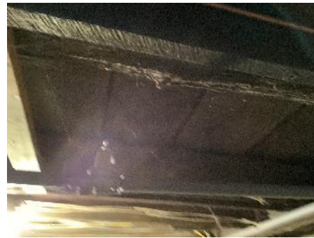
#11 – There is no insulation between the floor joists in the basement. Mineral wool batts would be a good solution.
