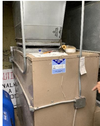
H4 – This hydro-air unit runs hot water from the boiler through an air handler to blow warm air into the Sanctuary.
