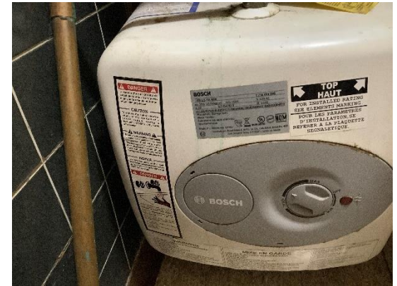
H-17 Point of use water heater
