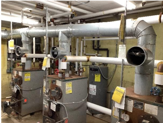
H1 – Three oil-fired boilers provide the bulk of heat to the building.
