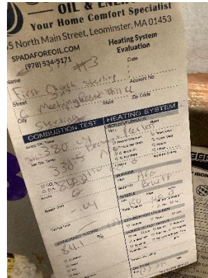
H-3 – A recent service measured actual efficiency as 84.1%, indicating the boilers are in good condition for their age.
