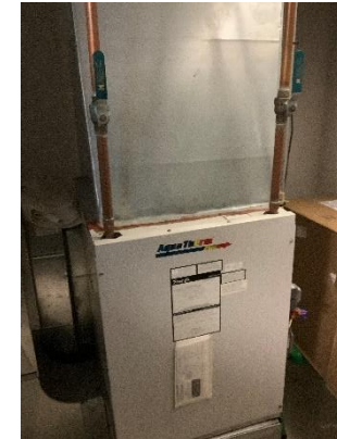
H5 – This hydro-air unit serves the basement
