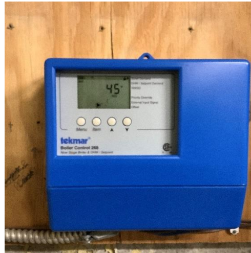
H9 This Tekmar controller provides outdoor reset and boiler sequencing capabilities.
