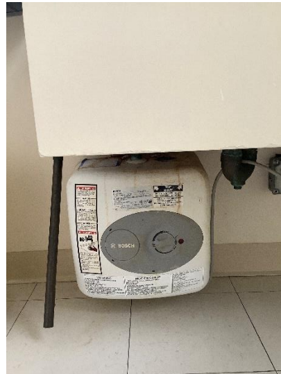
H-16 Point of use water heater
