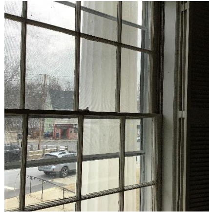
BE9 - Sanctuary windows are double hung with sash weights. Weatherstripping can cut down of air infiltration.
