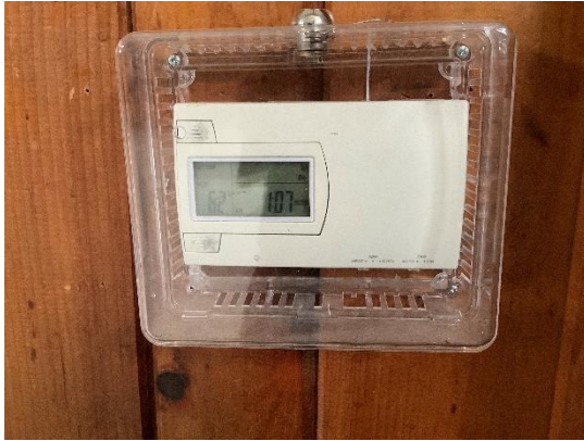
B1: Tstat 1 – Parish Hall
