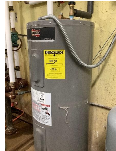
H11 This electric 40-gallon hot water heater dates to 2015, as indicated in the label in Photo H-2
