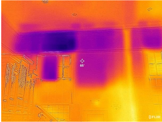
BE1 — Infrared photos of the Sanctuary walls show dark areas of missing insulation...
