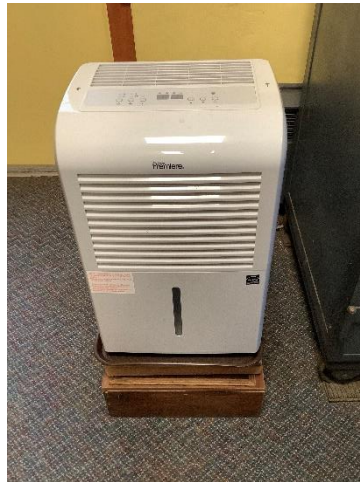
E8 - Dehumidifier in Choir Room
