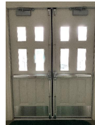
BE12 - The church doors are relatively new and tight fitting, though there are small gaps at the top and bottom where light and air enter; try to fill these gaps.
