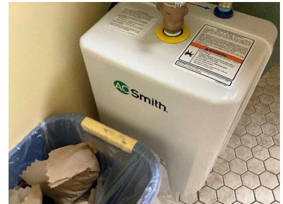
H-18 Point of use water heater
