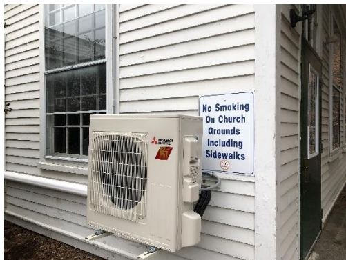
H8 – The new Mitsubishi heat pump that serves the Houghton Room.
