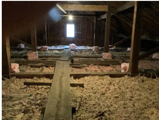
BE3 — The Sanctuary attic has about 10 - 12 inches of blown insulation; more could be added.
