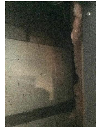
BE6 — A gap was left between the foundation wall and the insulation, seen through a hatch in the wall in B4.
