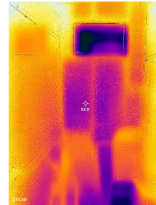
BE5 — Infrared photo of wall in Room B4 shows heat loss despite insulation.
