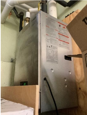
H13 – This propane-fired on-demand hot water heater serves the kitchen
