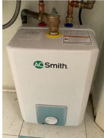
H- 15 Point of use water heater
